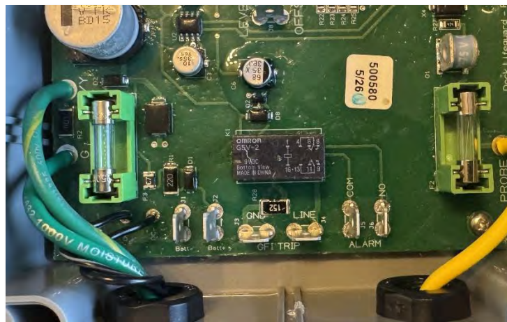
Figure 14, Voltage Surge Protection Fuses
